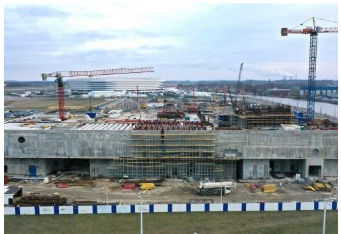
Construction of the Cultural and Educational Centre is under way in Kaliningrad. Photo /the Kaliningrad region government website
